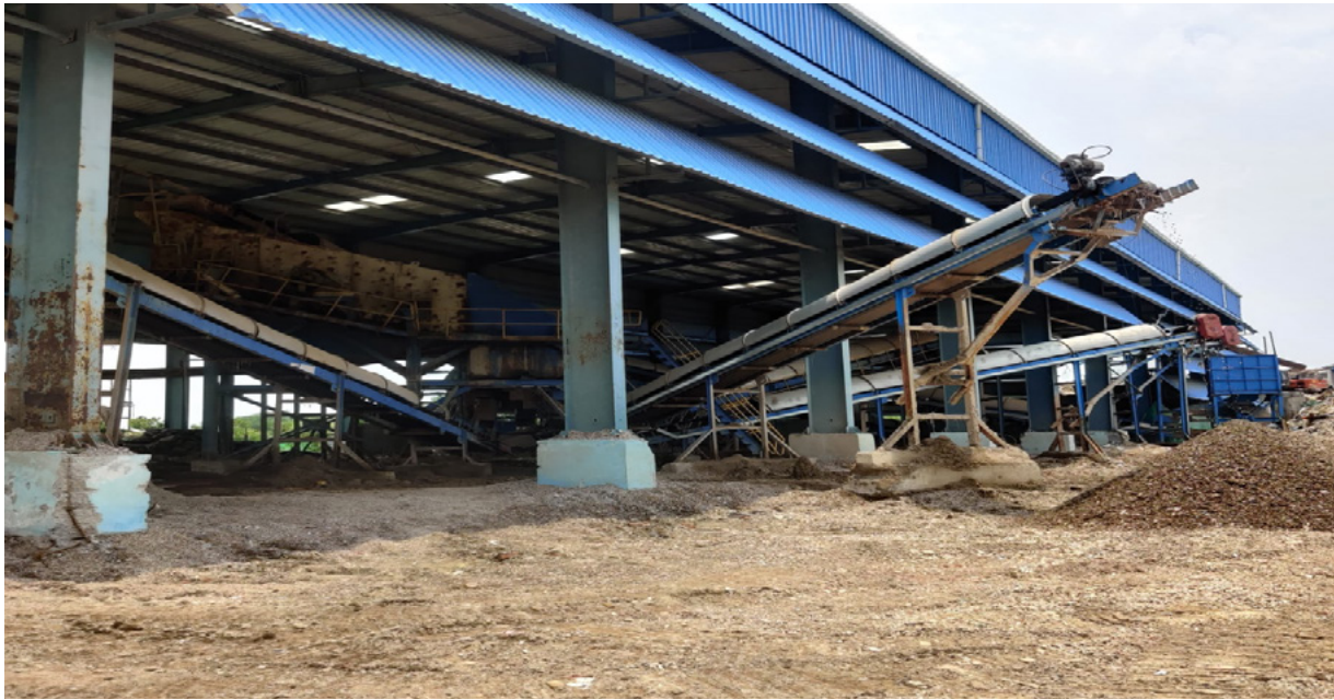
Figure 14-: Noida C&D Waste Recycling plant
